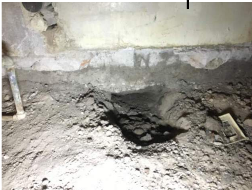
Unreinforced concrete footing with bottom inches below grade
